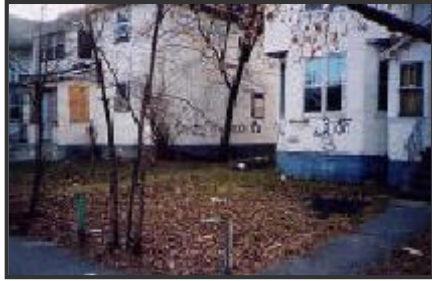
(Deteriorating Young Street Housing WBDC 2004)
